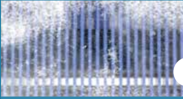
outdoor unit frosting
